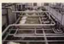
Wastewater Treatment Plant
